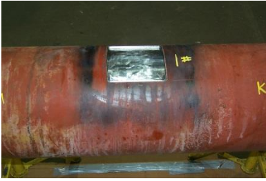
Defect - 6.5" x 6.5" x .300" Deep
