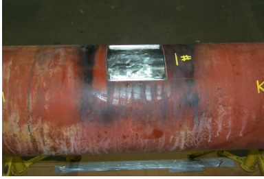
Defect - 6.5" x 6.5" x .300" Deep
