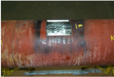
Defect - 6.5" x 6.5" x .300" Deep
